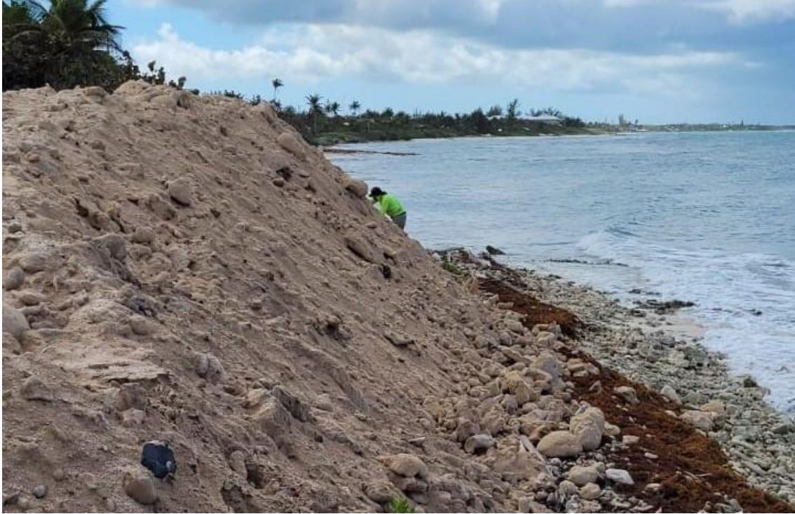
Figure 13: Material stockpiled too close to the water's edge which would or would be likely to enter the marine environment during a storm.
