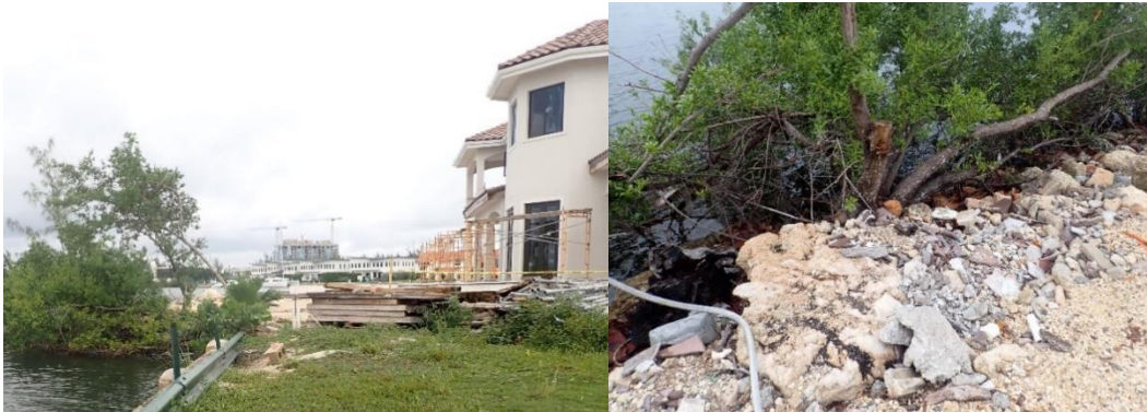
Figures 7 and 8: Loose materials and construction debris being stored on the canal side of a development, and that material entering into the marine environment.
