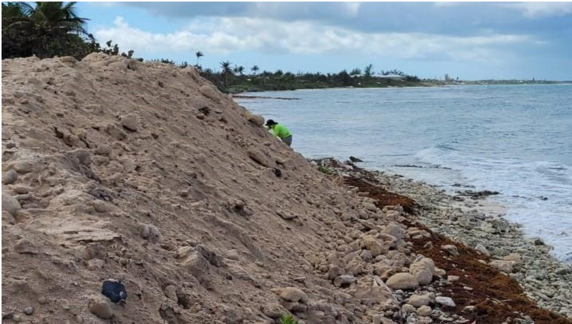
Figure 11. Material stockpiled too close to the water's edge which would or would be likely to enter the marine environment during a storm.
