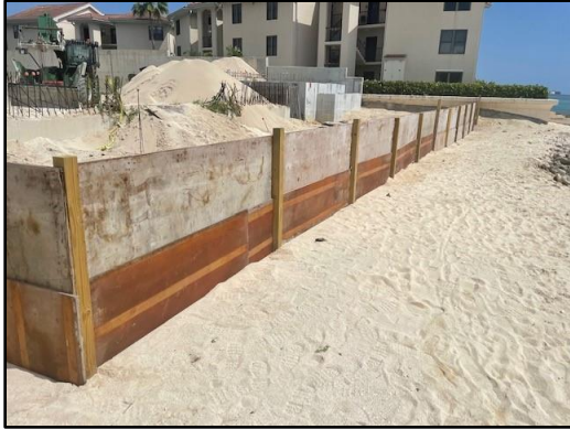
Figure 6. An example of suitable construction fencing to protect turtles (Source: DoE, 2022).
