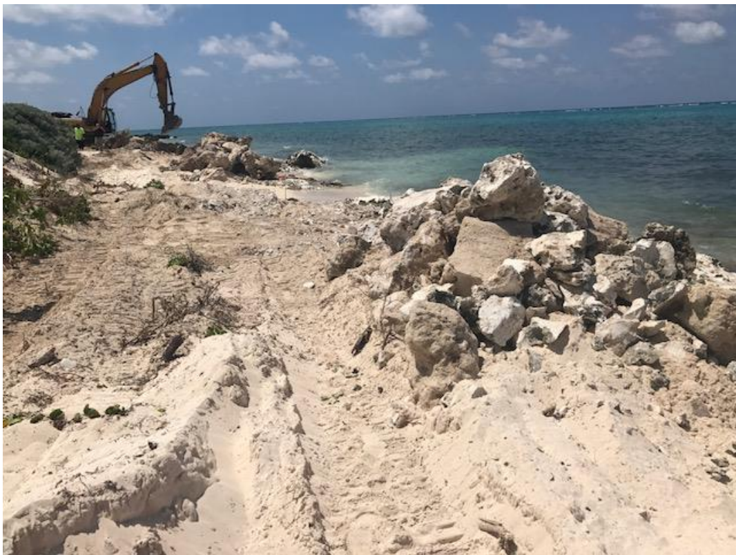
Figures 6 and 7. The DoE responded to a complaint from the public that this stockpiled material was causing considerable turbidity and siltation of the marine environment.
