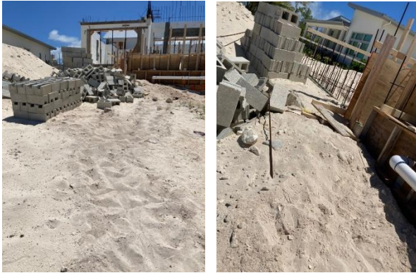
Figures 4 and 5: DoE photos showing turtle tracks within a construction site on a turtle nesting beach. This site did not have temporary beachside construction fencing to prevent turtles from entering the site. The turtle could have or may have been injured by construction materials and debris on-site (Source: DoE, 2023).
